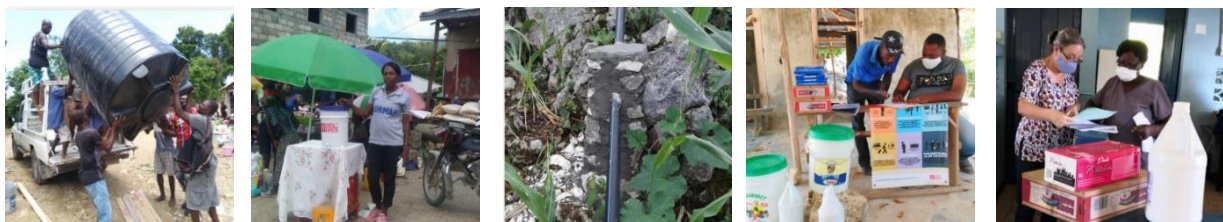
78 water points with tanks and 800 hand-washing stations installed, and Rehabilitation of water infrastructure to secure access to water.
